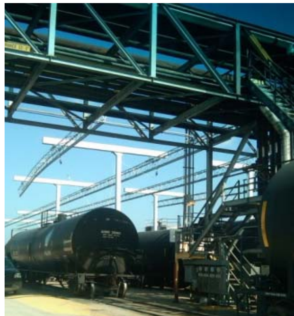
Figure 7: Retrofit of Overhead Support Beams for Attaching Safety Lanyards to Access RC Domes
