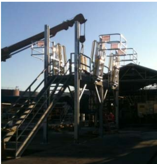
Figure 12: Crane Lowering New, Pre-Fabricated Fall Protection Platform for a Truck Rack Into Place
