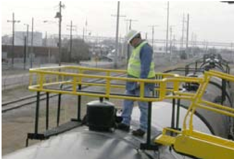
Figure 6: New Rail Gangway and Cage
